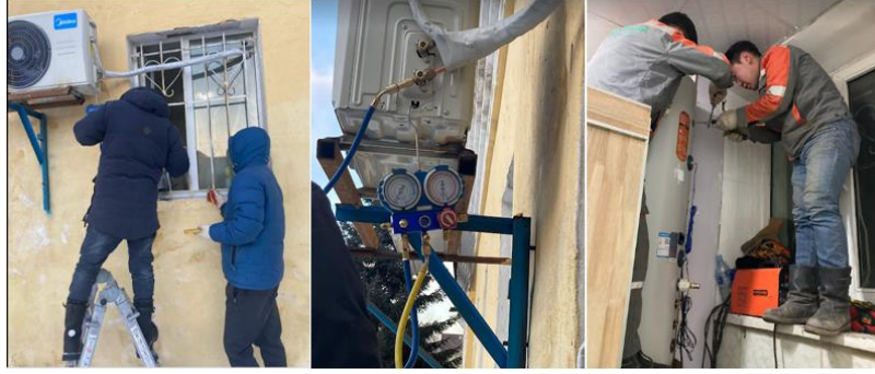
Fig. 2. Installation and setup of the air-to-water heat pump domestic hot water system
